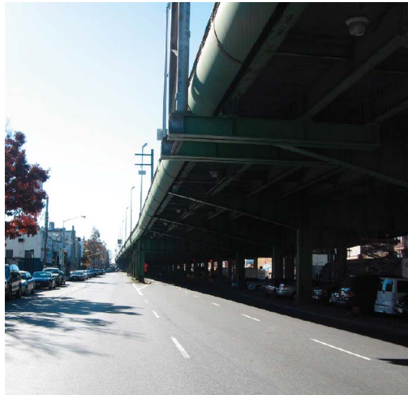
The elevated Gowanus Expressway over Third Avenue is a major visual, physical and psychological obstacle to people circulating freely around the community of Sunset Park.
